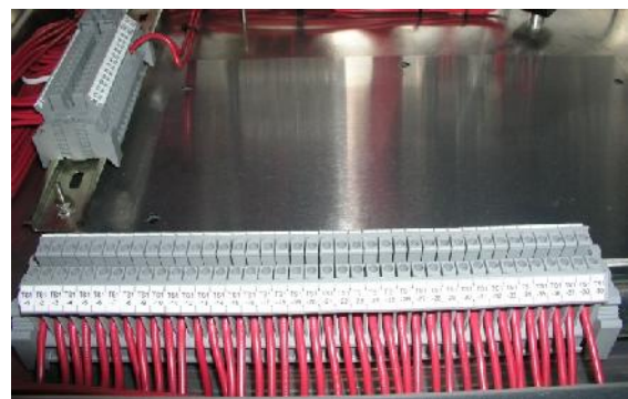
View showing easily accessible terminal blocks.
